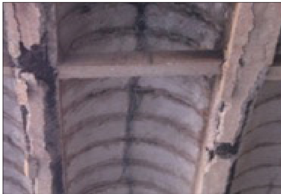
Signs of Deterioration after 50 Years
